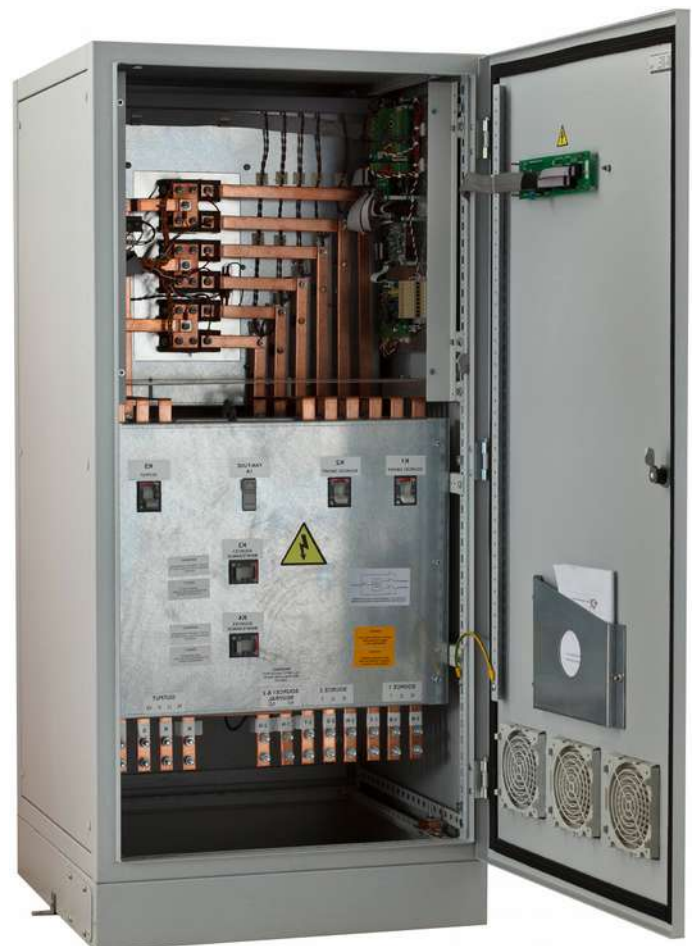
Static Transfer Switch STS Internal View
